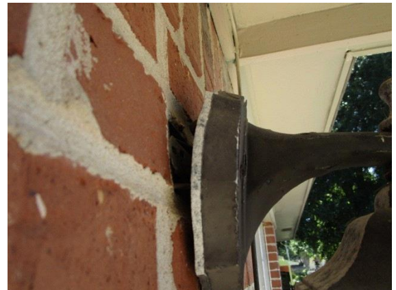
Light fixture separating with exposed wiring.
