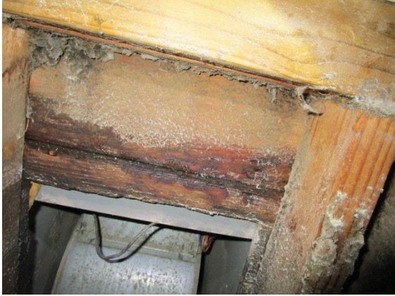
Active leak into plenum
