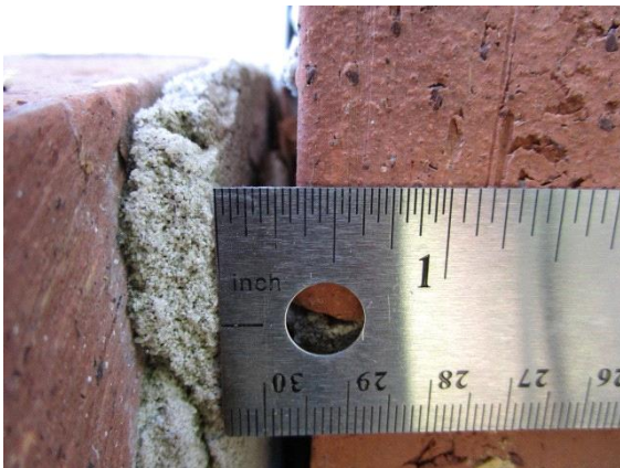
Bedroom window sill with signs of separation.
