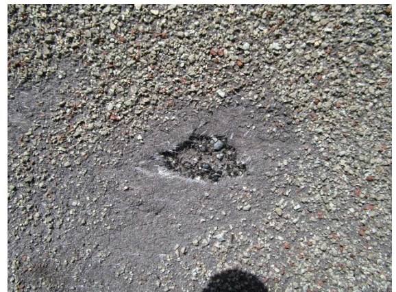
Hole with granular loss. Possible hail damage.
