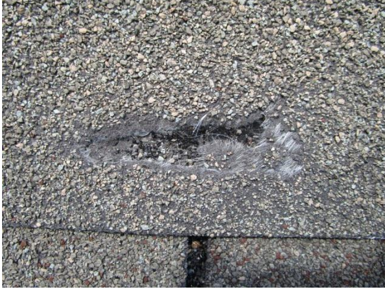
Hole with exposed fibers.
