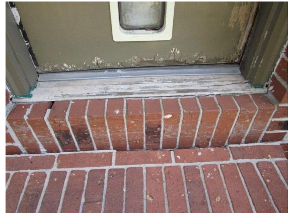
Exposed/moisture damaged wood.
