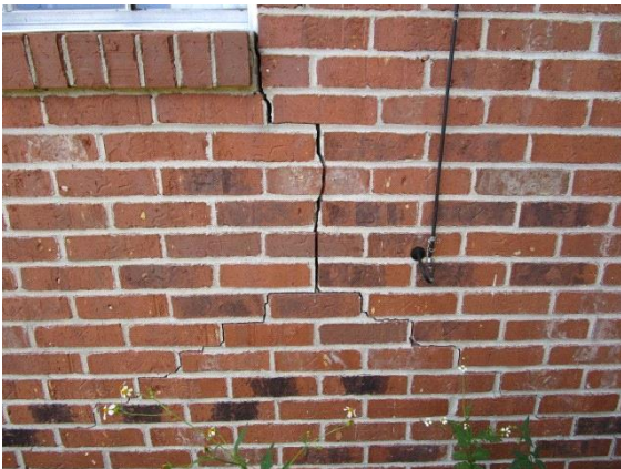
Bowing and cracks.
