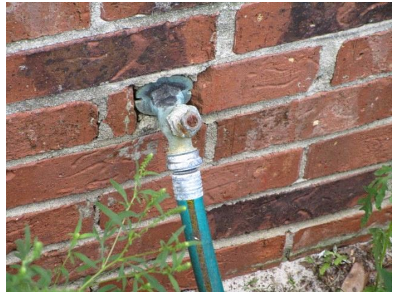
Missing hardware. Unable to test.
