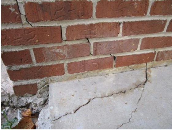
Cracks in concrete and brick.
