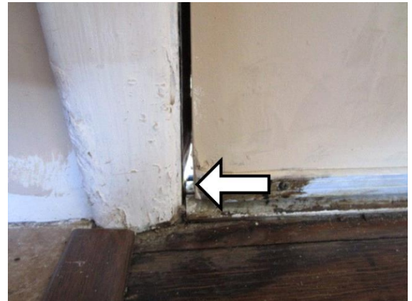
Air leak, back door.
