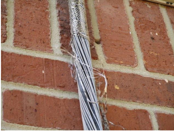
Service line sheathing heavily weathered.
