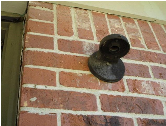
Backlight exposure, missing light/cover.
