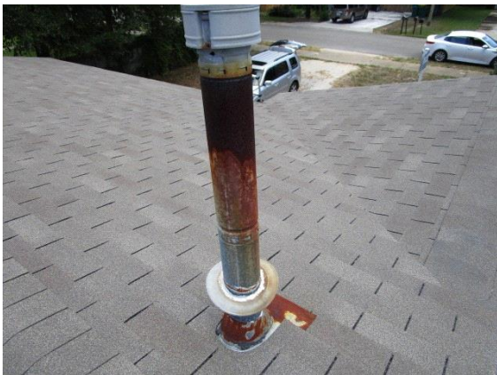
Rusty flue with failed caulk bead
