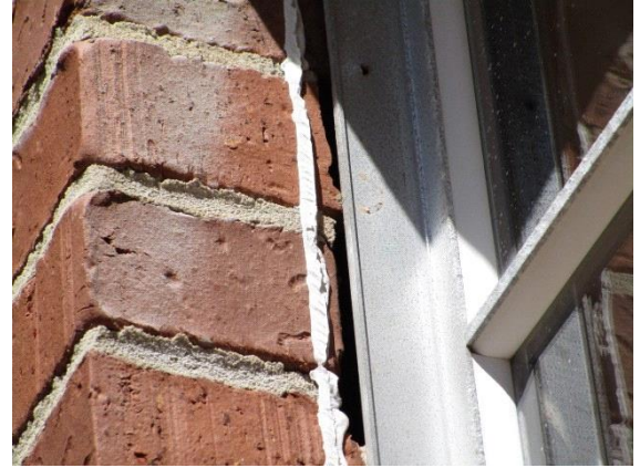
Window frame/siding separation.
